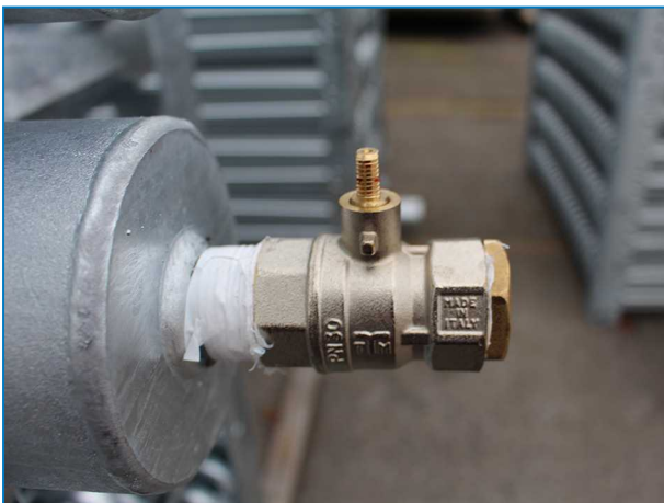
Upper coil connection with pressure release valve on condensers.
