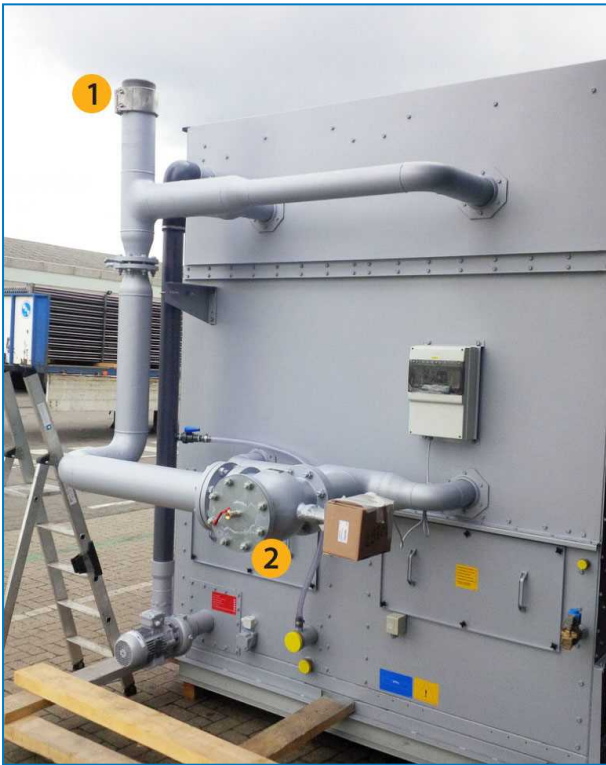
Unit with closed external piping
